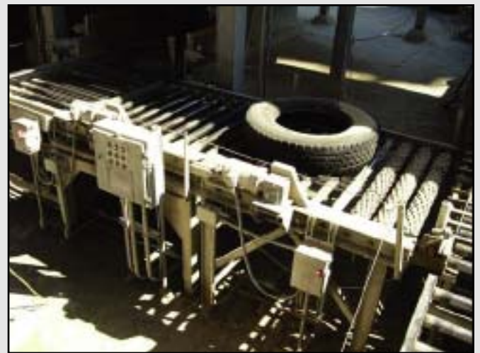
Each tire is weighed to allow the plant's control system to fine tune kiln operational parameters.
